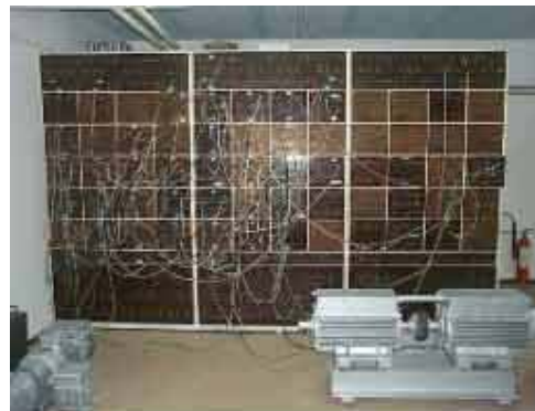
b) Connection panels
