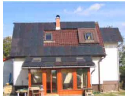
Grid Interactive solar house, 2.6 kWp Installed power
